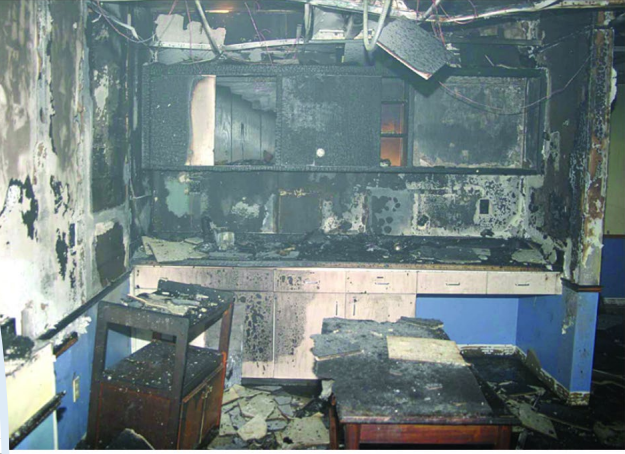
3 a kitchen. Note the V pattern of burning on the wall on the left side. Courtesy of James Novak.
